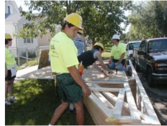
Dean Thomas, Habitat homeowner of the Eastview house, working on trusses in July.
