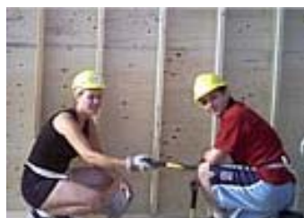
Two members of the Interfaith Youth Build work on the house at 433 Langside St.
