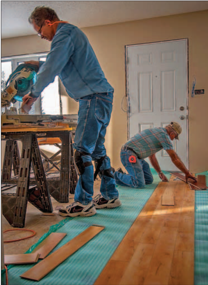
Habitat for Humanity volunteers lay flooring in the recently completed Virden home. (Photo courtesy Vaughn Bender)
